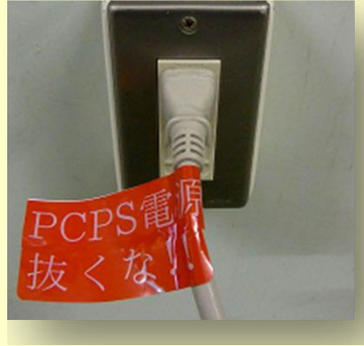
Fig. 2 (Red caution tape indicating "DO NOT UNPLUG")
